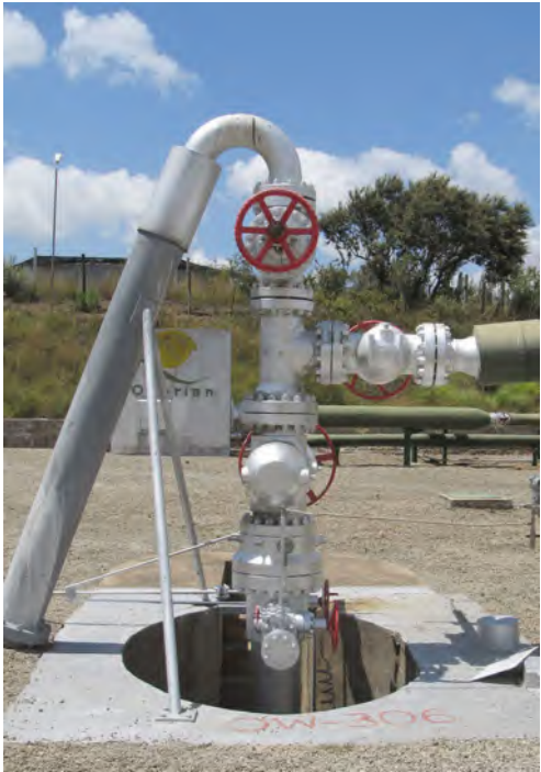
Figure 3.9: Deep geothermal wellhead ©Sanjack Petro
